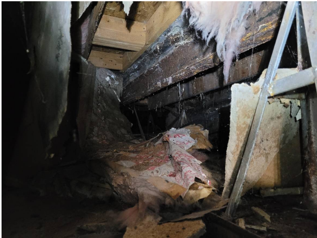
Figure 4 – an area near the entrances where the wood joists have considerable deterioration.
