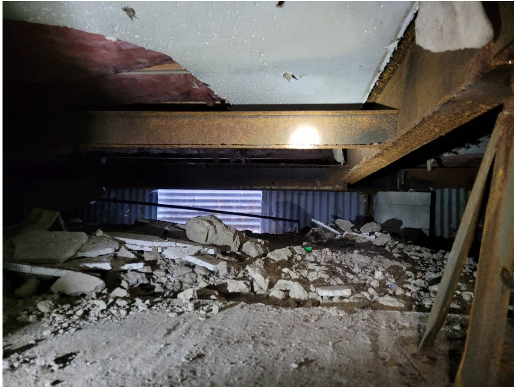
Figure 3– another area close to an entryway with considerable corrosion.
