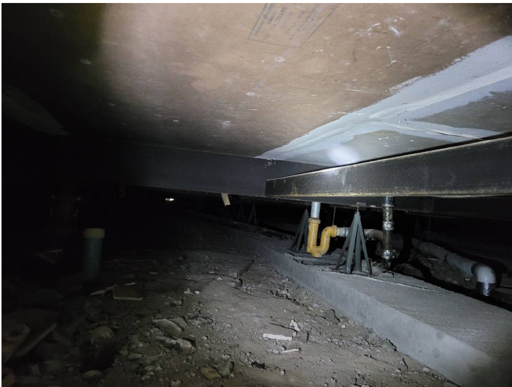
Figure 2 – an area away from the entrances where the steel framing and jack supports are in considerably better condition, though some light corrosion is observable in the top and bottom of the steel beam to the right.
