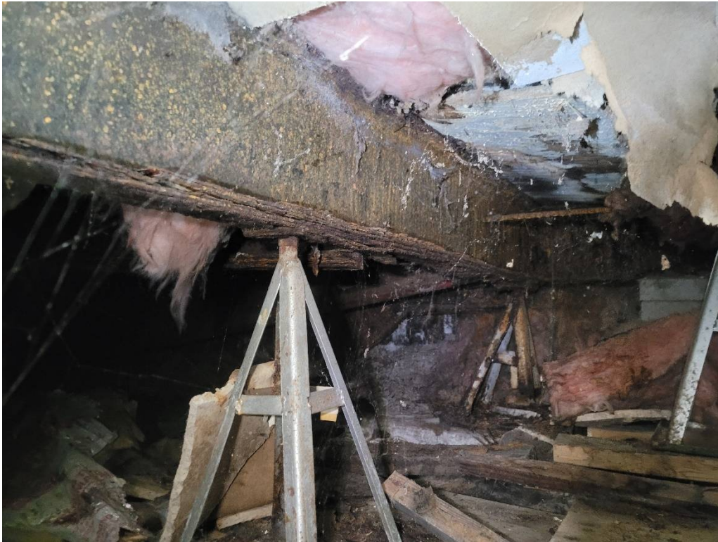
Figure 1 – steel jack supporting a steel beam, both of which have considerable corrosion. The wood framing above is unobservable, though the damage to the sheet rock may indicate water damage to the wood framing as well.
